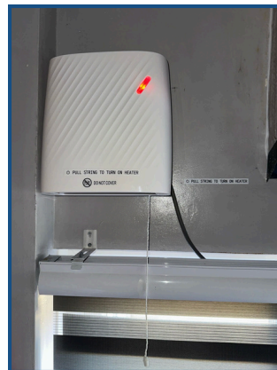
Spa Room Heater
