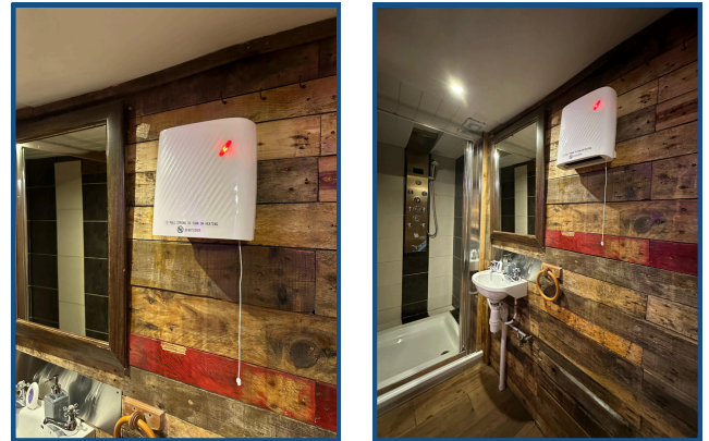
Spa Room Heater
